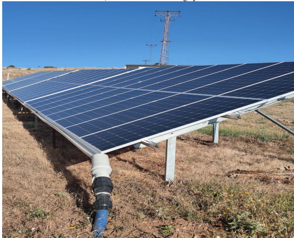
b) PV array and water collection channel
