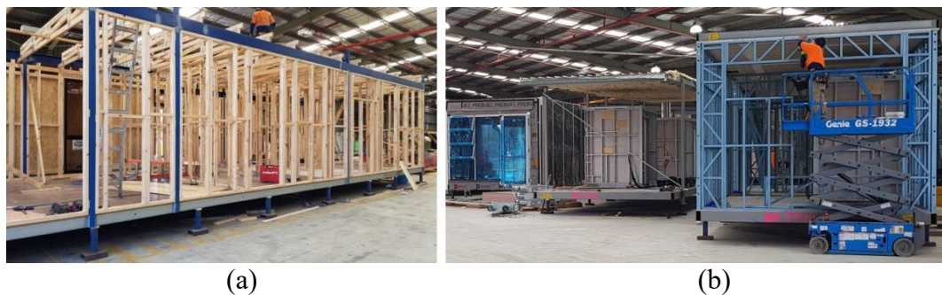
Figure 1. (a) Wooden wall system inside a steel-framed modular unit, (b) modular structure created with light steel structure (Gunawardena and Mendis, 2022)
